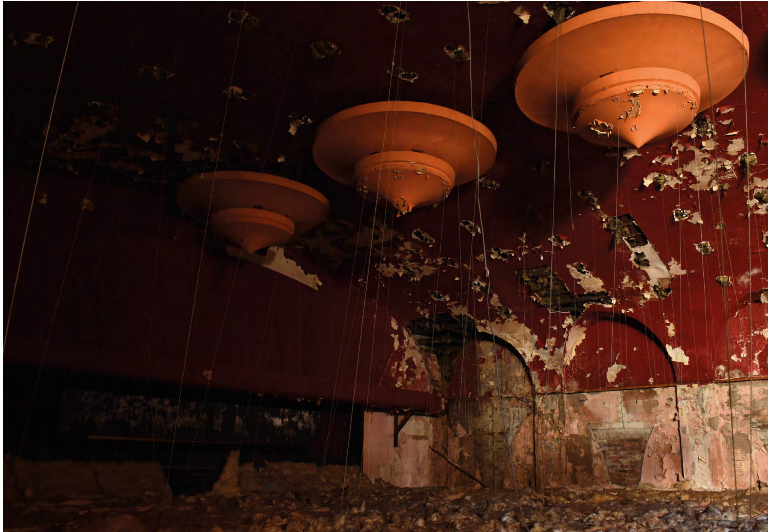
The roof of the cinema that is to be salvaged (D Meurig 2021)
