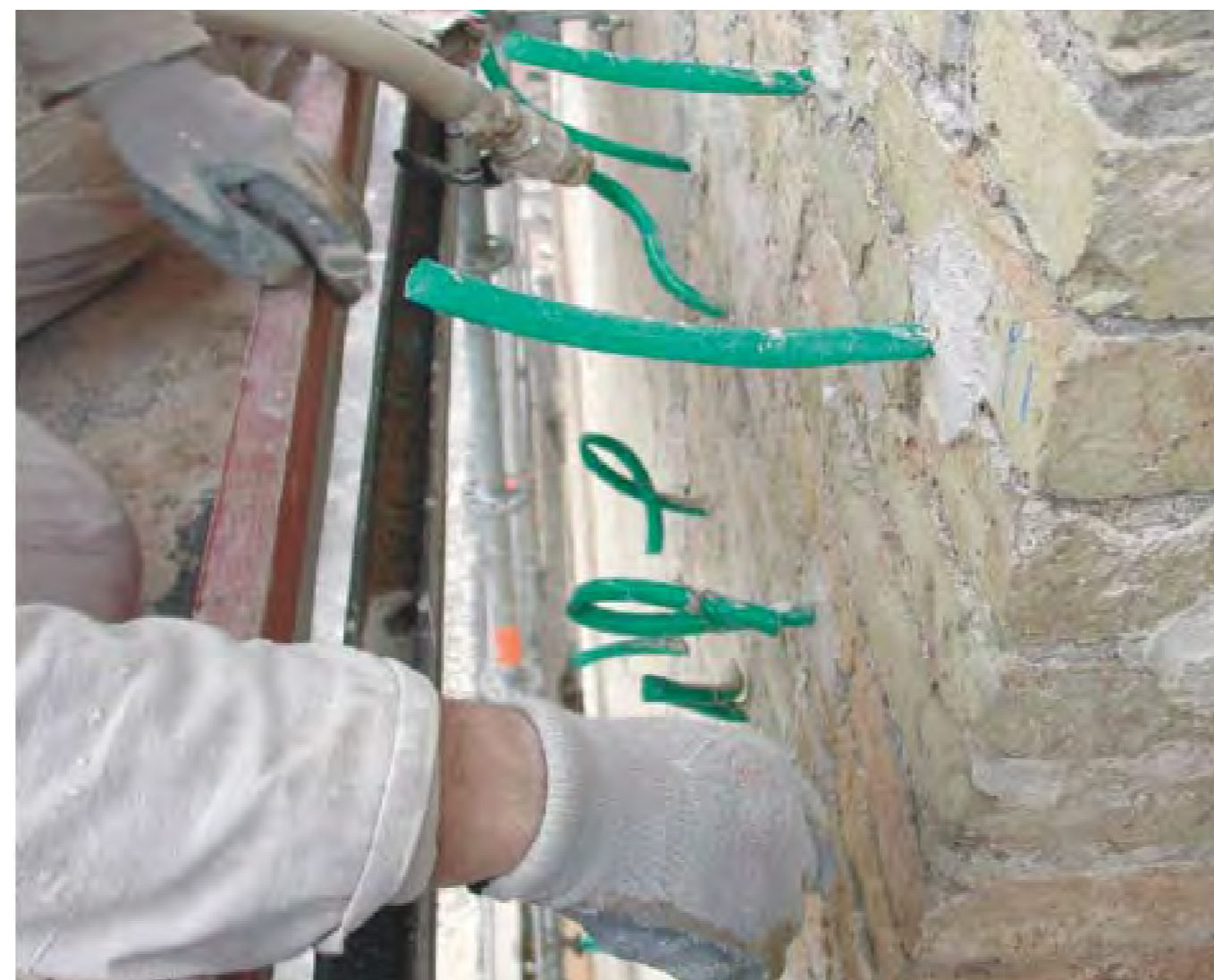
Injections to strengthen the walls may be necessary in certain places (Modena et al 2011).
