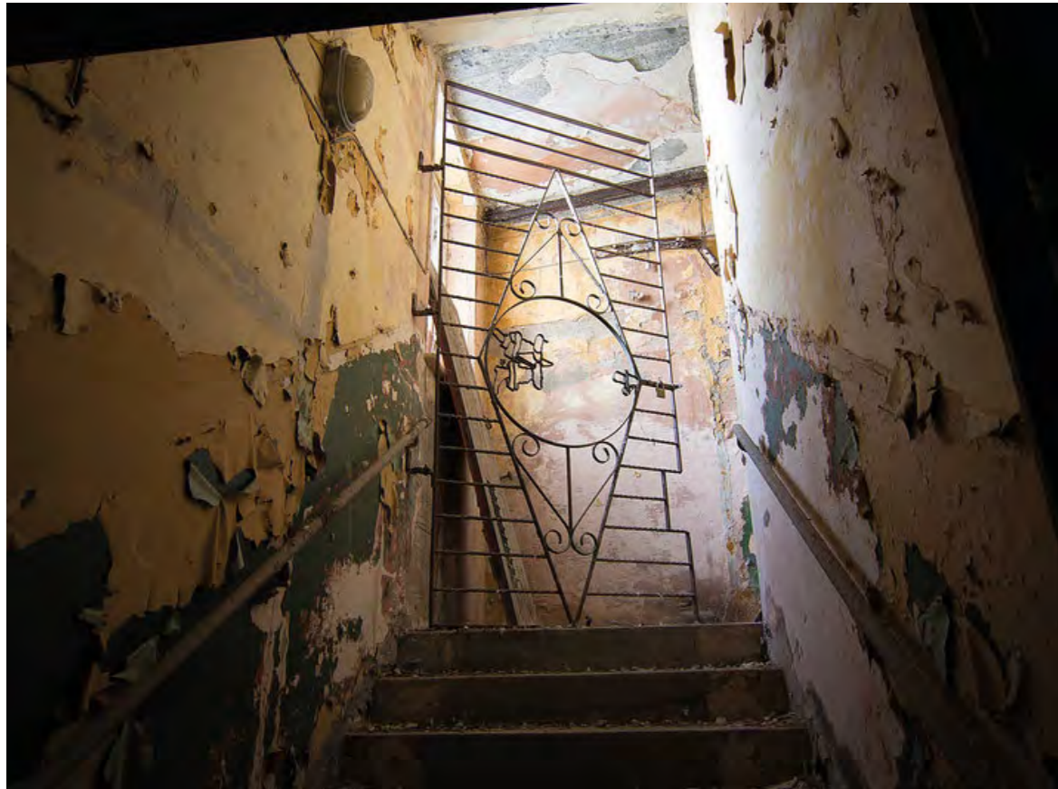
Detached stairwell gate (Lenston 2015).
