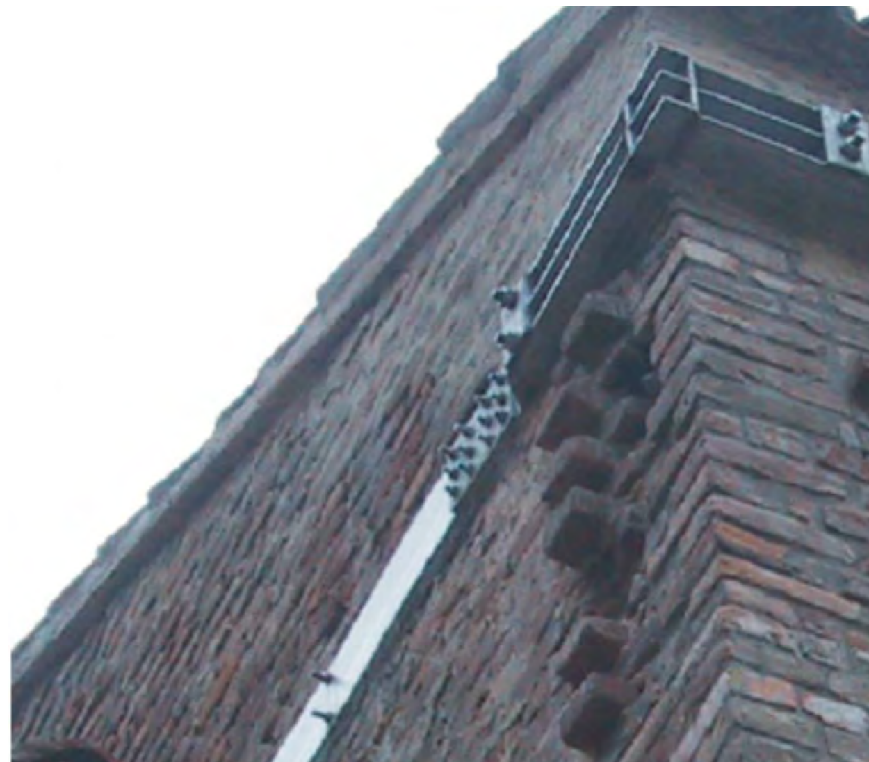
Steel plates will be used to strengthen the wall and connect it to the timber elements (Modena et al 2011).
