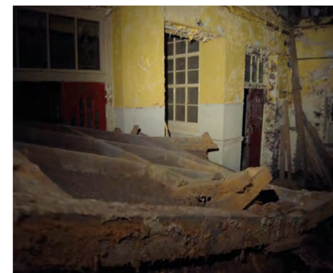
4. Concrete steps to the basement reveal a portion of the ceiling that has collapsed. To access the Labour club and conference halls it must be ducked under.
