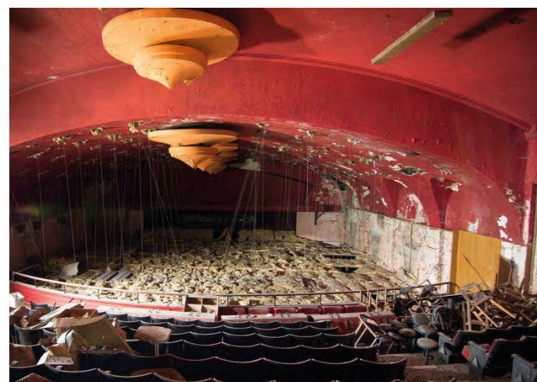
2. The steps of the upper seating area are falling through in parts. The sunburners on the ceiling provided light and ventilation. A false ceiling was suspended to increase thermal efficiency. There is currently little access to light.
