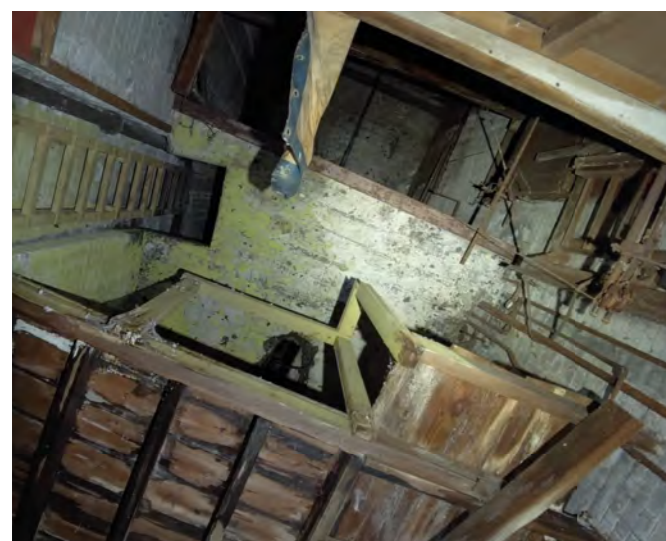
1. The fly tower houses the stage and layers of internal structure, all of which is unstable.
