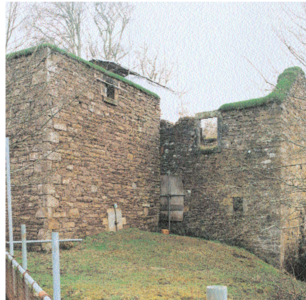
Earth capping was considered for the wall but deemed unnecessary (Historic England 2013).
